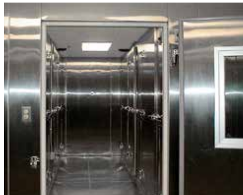
Typical hall access to multiple cold storage compartments - stainless exterior
